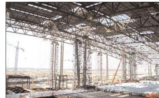
The view from inside the new 1.2 million-square-foot terminal structure on a space between existing runways that continue operating during construction.
