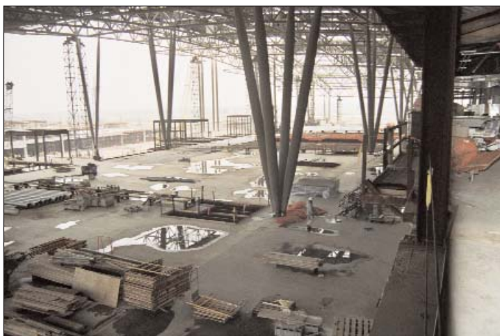
The IPS strategy was to be ready to be the first to move into each completed space, and begin hanging their pipe right away. It enabled them to install large-bore pipe early in the project
