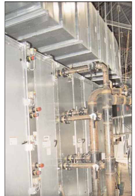
Air handlers had to arrive inside the terminal before the walls were up. They were set around the building using various processes.
