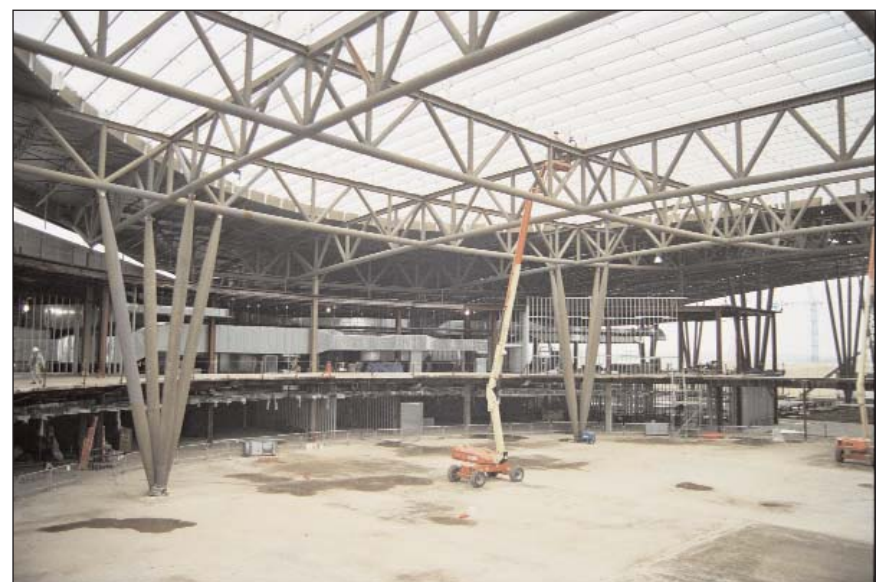
Workers install the transparent roof panels inside the terminal's Civic Plaza area. This area's final phase was installation of radiant heating and cooling piping cones on top of the sub-floor. Once tested and approved, the multi-zone system was covered with a concrete slab and Terrazzo coating.
